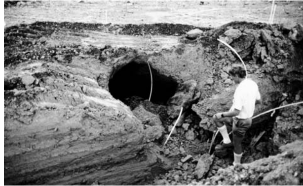
Figure 7. Internal erosion in the dam core
