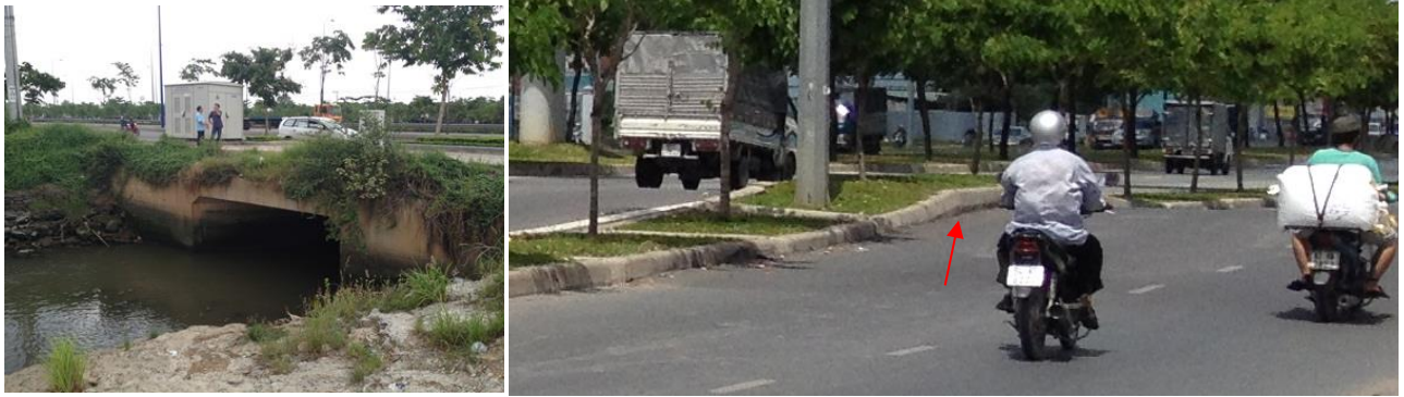
Fig. 4.1 Concrete culvert and unequal settlement on road surface (Hochiminh City)
