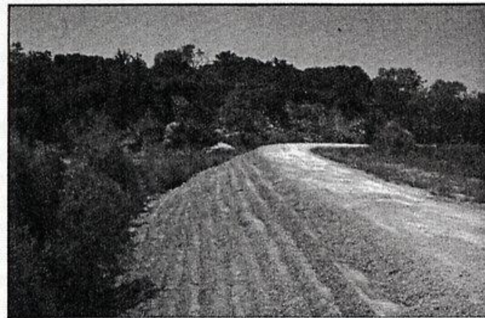
Figure 4. RCC overlay at Brownwood Country Club Dam after several overtoppings.
